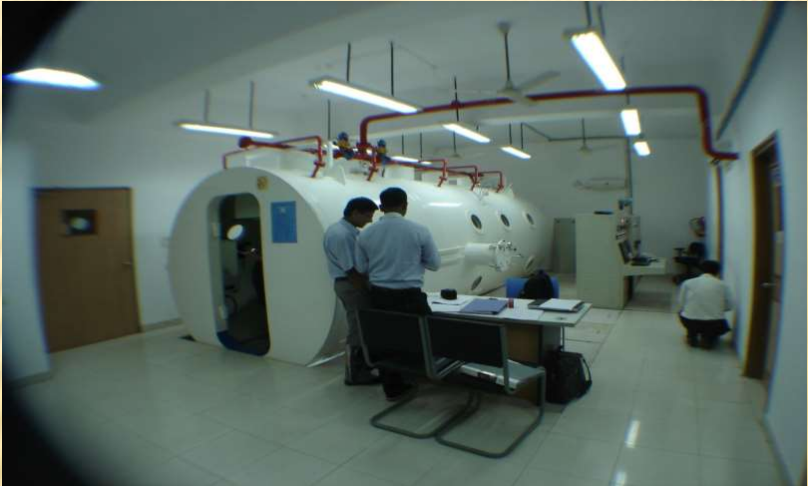
HBO CHAMBER AT GODREJ HOSPITAL , MUMBAI
